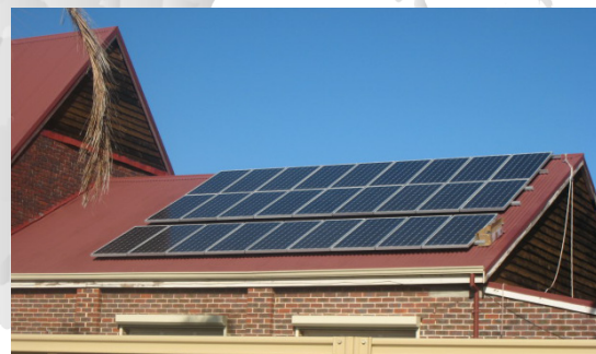
Location : Perth, Australia Construction type: Residential rooftop Completion date: 2012 Operator/installer: Phase
