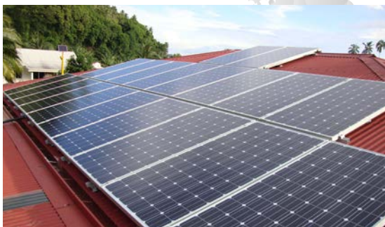
Location : Various cities, French Polynesia Construction type: Residential rooftop Completion date: 2012 Operator/installer: Conexun
