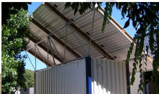
Location : Madagascar Rated system size: 3.8kW Construction type: Built-in PV container Completion date: 2011 Operator/installer: IE Solar
