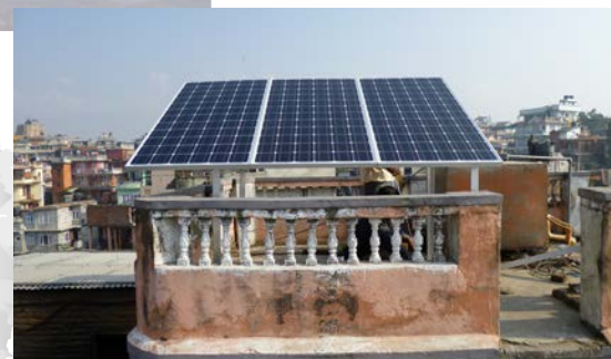
Location : Nepal Rated system size: 570W Construction type: Off-grid residential rooftop Completion date: 2012 Operator/installer: Solar Solutions
